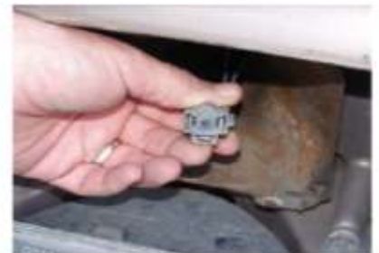
P15-6 Check the wire connector for corrosion or other foreign material. Clean as necessary.
